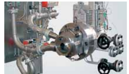
Process water piping
